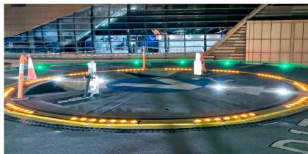
Above: Joby's GEACS charging equipment installed in the VDX vertiport at Dubai International Airport
